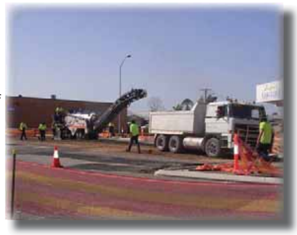
Right: A new roundabout was installed at the intersection to Tozer and Elbow Streets in West Kempsey.
