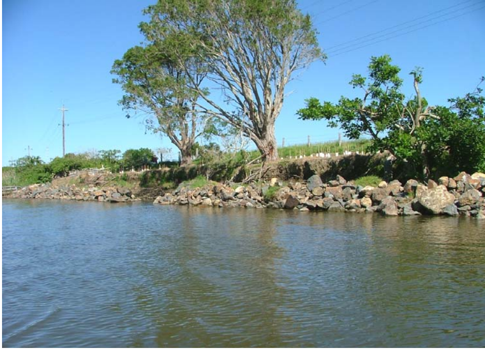
Voluntary Streamcare Grants Scheme Project on the Macleay River. Rock wave barriers, planting and fencing. (E – 0497278, N – 6569866) (ArcView Project # 10 and 14)
