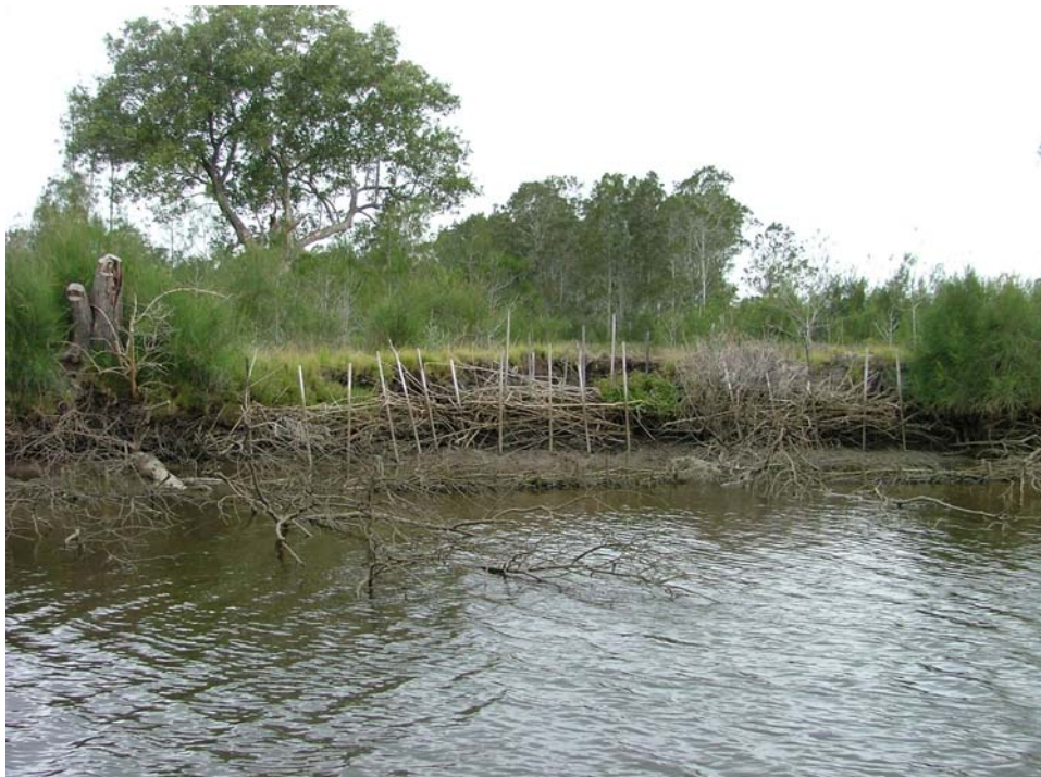
Voluntary Streamcare Grants Scheme Project. Brush groyne erosion control works along the bank of Clybucca Creek. (E – 0500000 N – 6578100)
