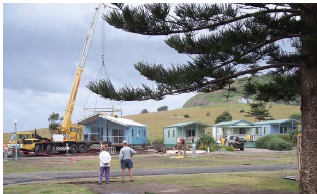
Right: New cabins installed at Crescent Head Caravan Park last October are starting to pay dividends.
