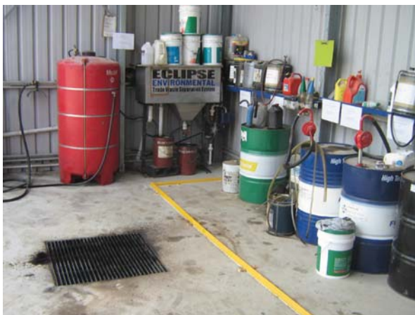
Example of site specific bunding installed which still allows unimpeded access to materials.
